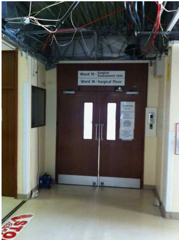
Figure 3. Photograph of the entrance to ward 16. The electrical cabling overhead was noted.
