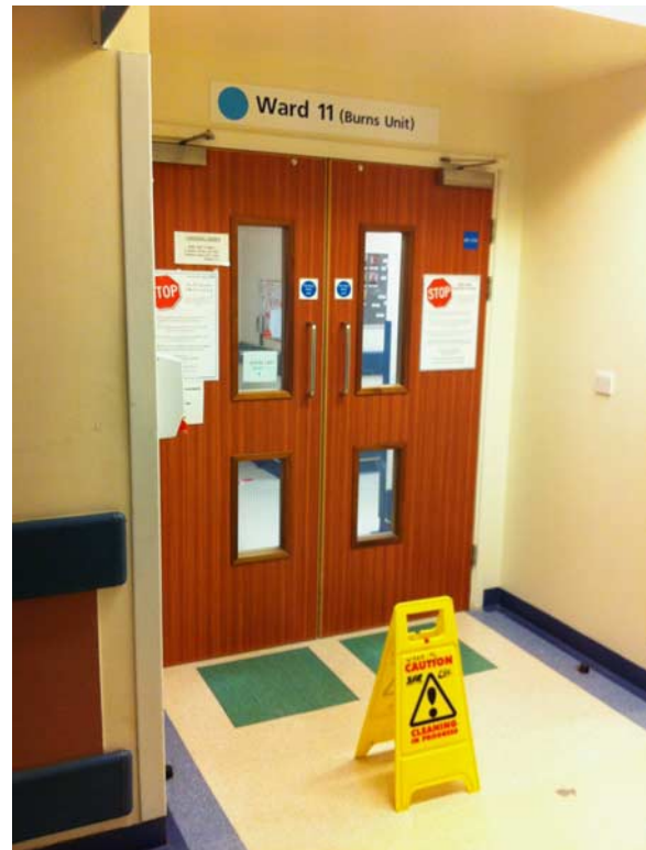
Figure 8. Photograph of the entrance to the Burns Unit. The Burns unit was not part of this study but a safety hazard in the form of a poorly placed "caution wet floor" sign was noted.
